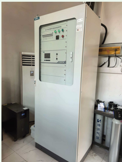
Online Monitoring Equipment
