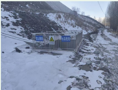
Newly Built Shaft Collection Tank and Diversion Channel
